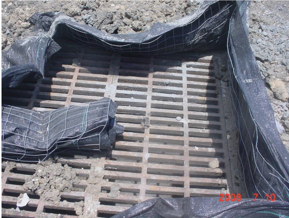
Poorly protected inlet
