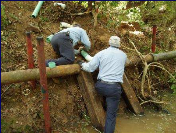
Broken sewer pipe
