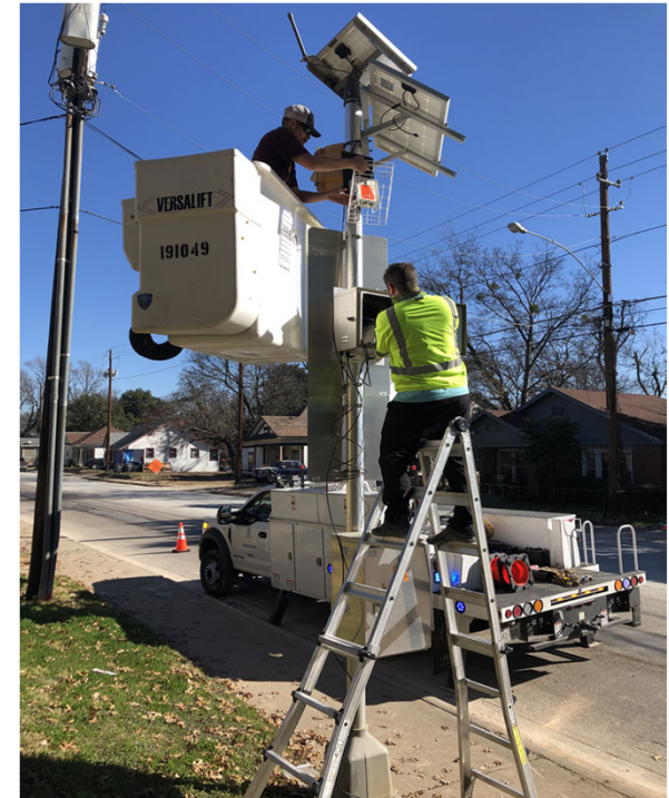
Air Quality monitor installation at Exline Recreation Center
